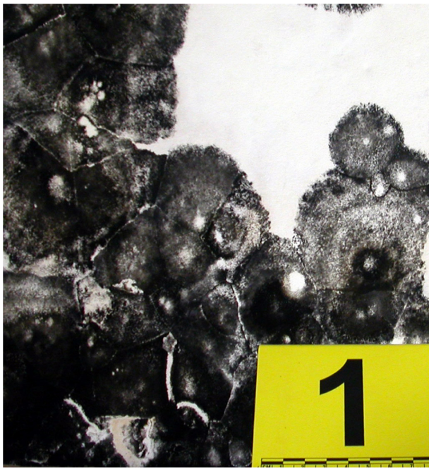
Figure 4 Colonies of Stachybotrys chartarum , the so-called “toxic mold”, developed on a vertical plastered wall affected by rising damp.
